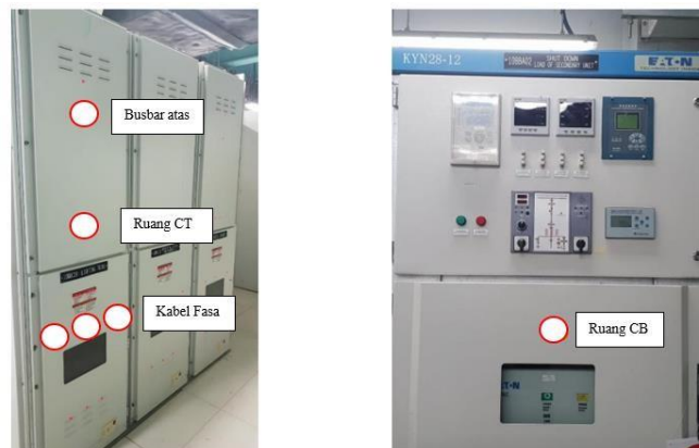
Figure 4. PD testing position.
