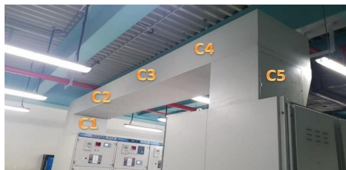
Figure 5. PD test location on a bus duct using the TEV and Ultrasound methods.
