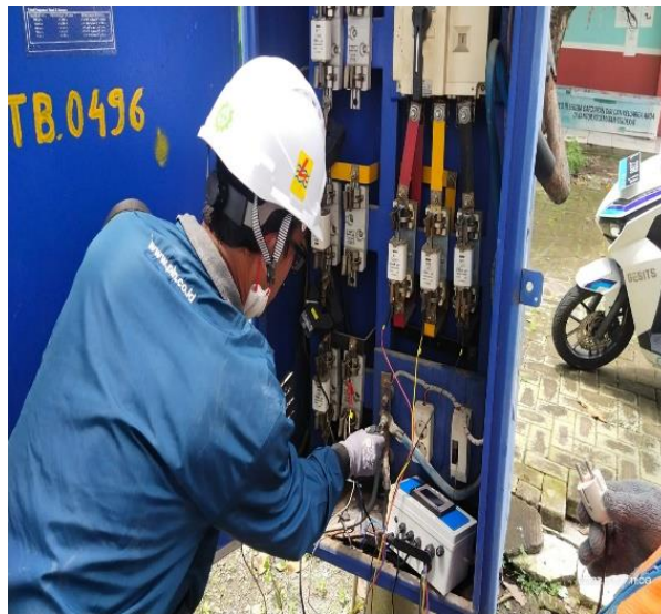
Gambar 6. Instalasi alat monitoring online di Site PLN UP3 SBS.
